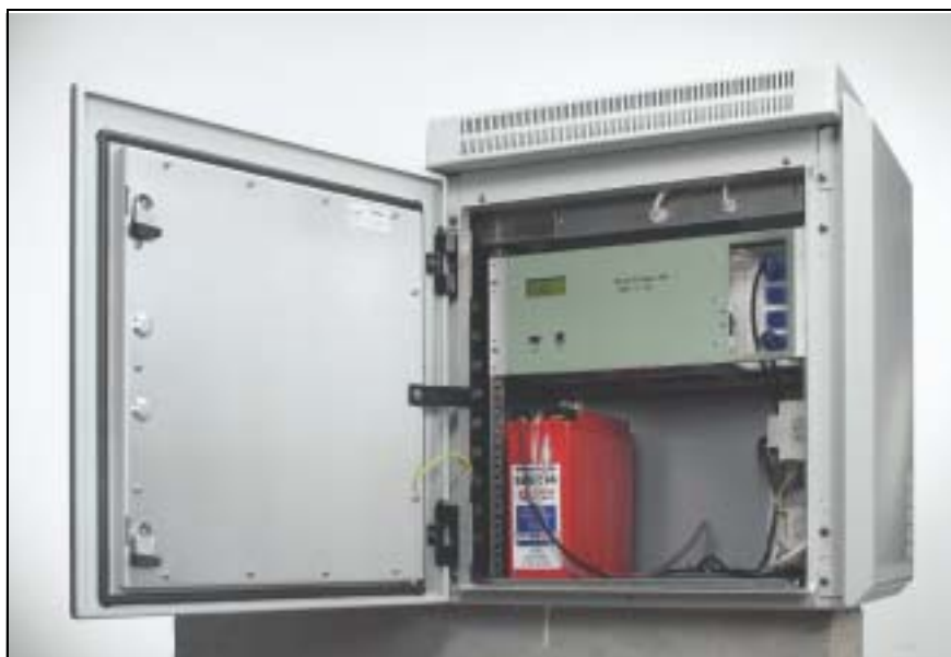
Fig. 2 Interior view of the weatherproof cabinet showing the position of the units. The basic Type 3597 C-001 System Unit is seen in the upper half of the picture. Noise Analyzer Type 4441 and Microphone Power Supply are included with the basic unit
